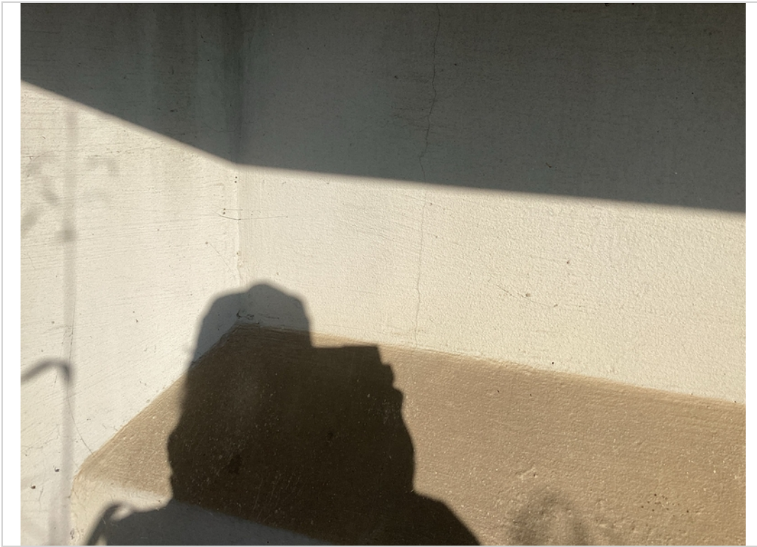
Beam E filler span 1 - Hairline crack (Typical all beams span 1&3)
