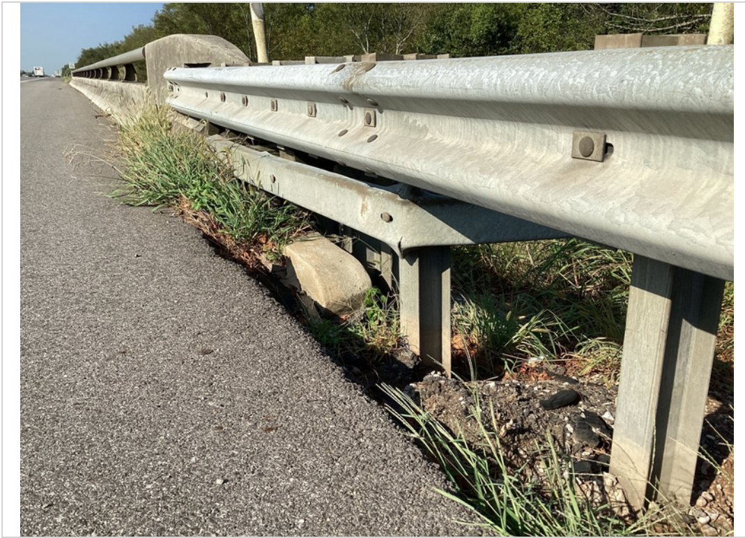
Approach 2 left transition rub rail - collision damage
