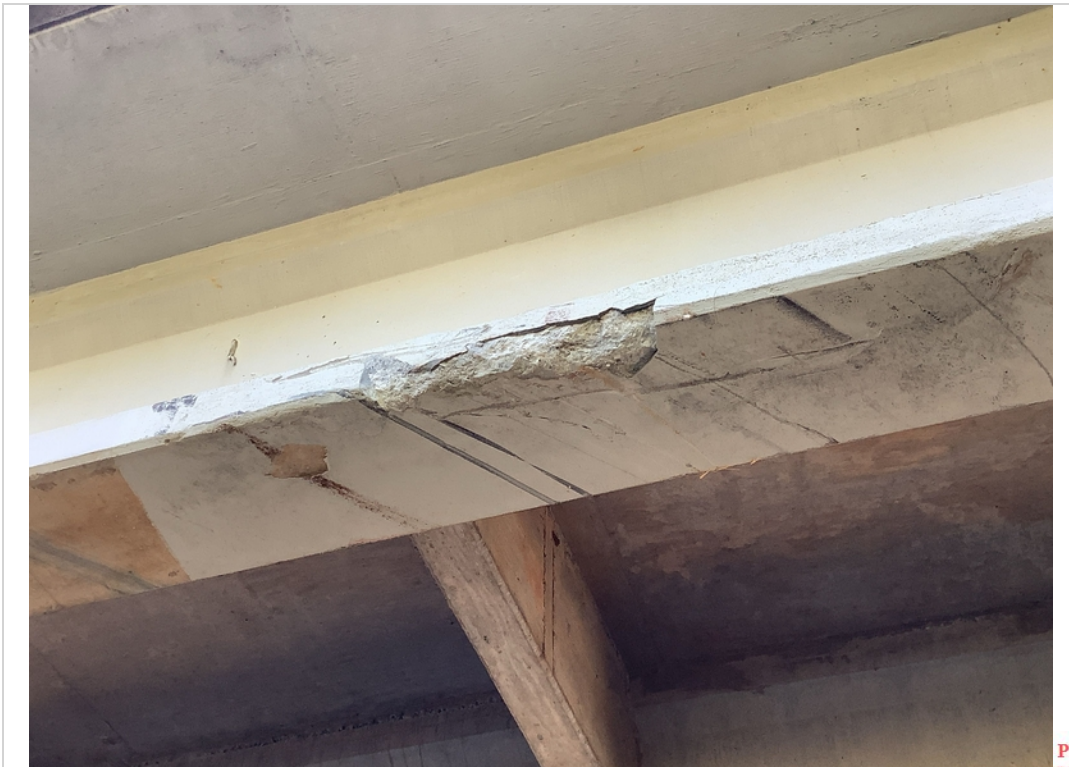
Span 2 beam A left side - spall (2' l x 6" w x 1" deep)
