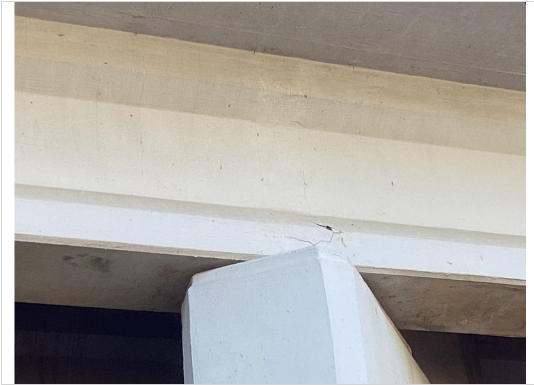
Beam A over bent 2 diaphragm filler - Hairline cracks (Typical other diaphragms over bents)
