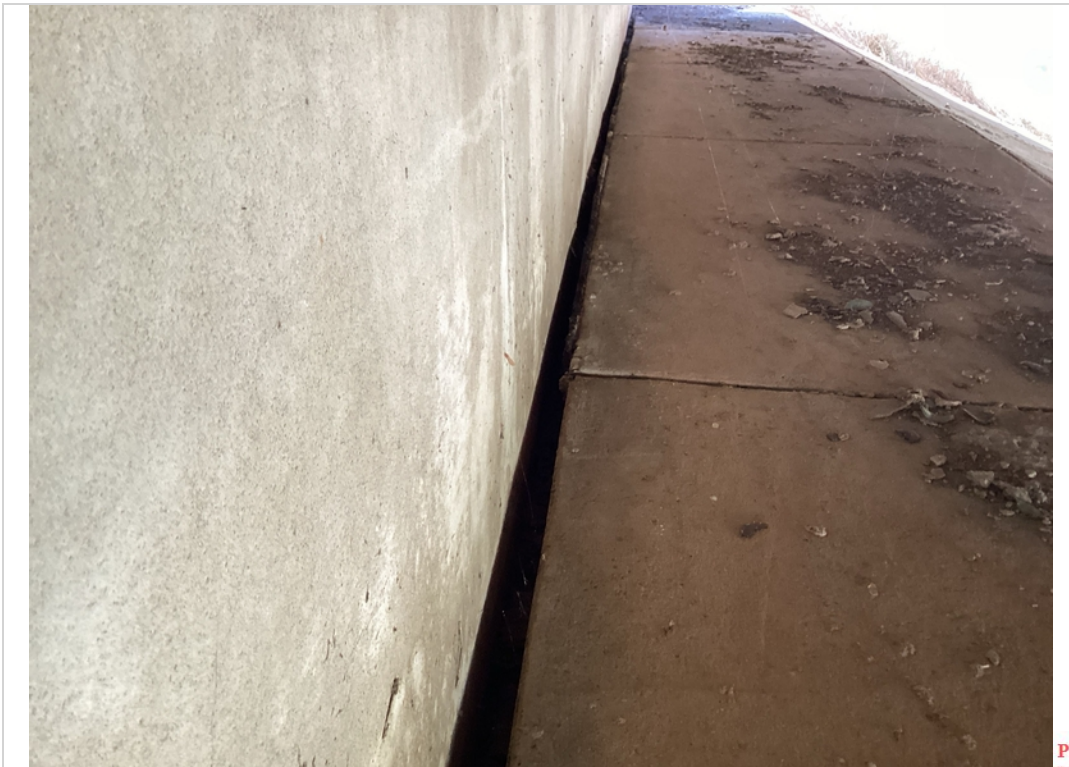
Abutment 2 slope pavement - " separation (typical)
