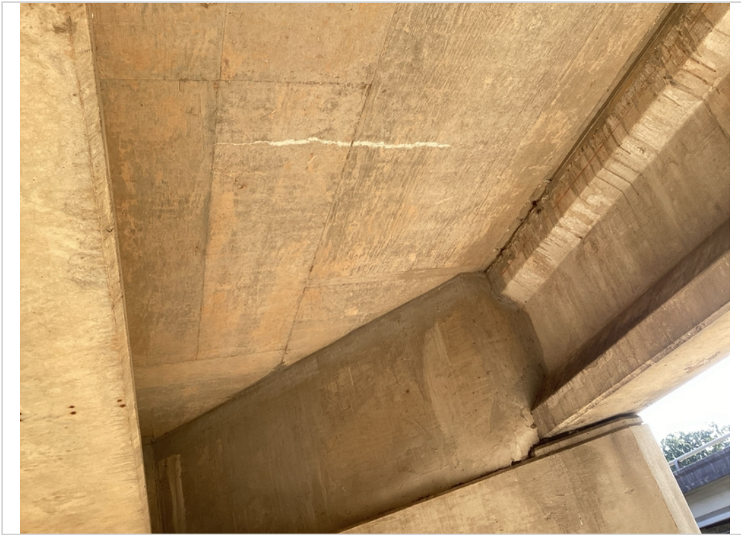
Bottom deck span 1 - Hairline cracks w/ leaching
