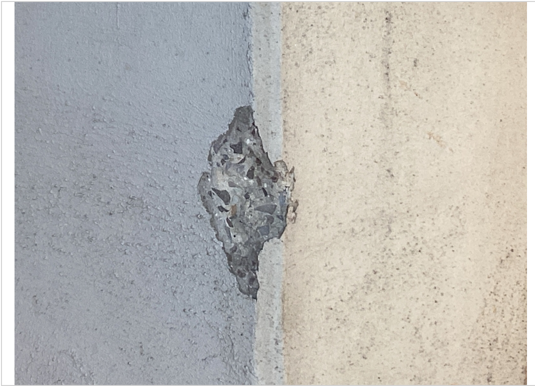
Bent 2 column B front - spall (6" diameter x 2"Dp)
