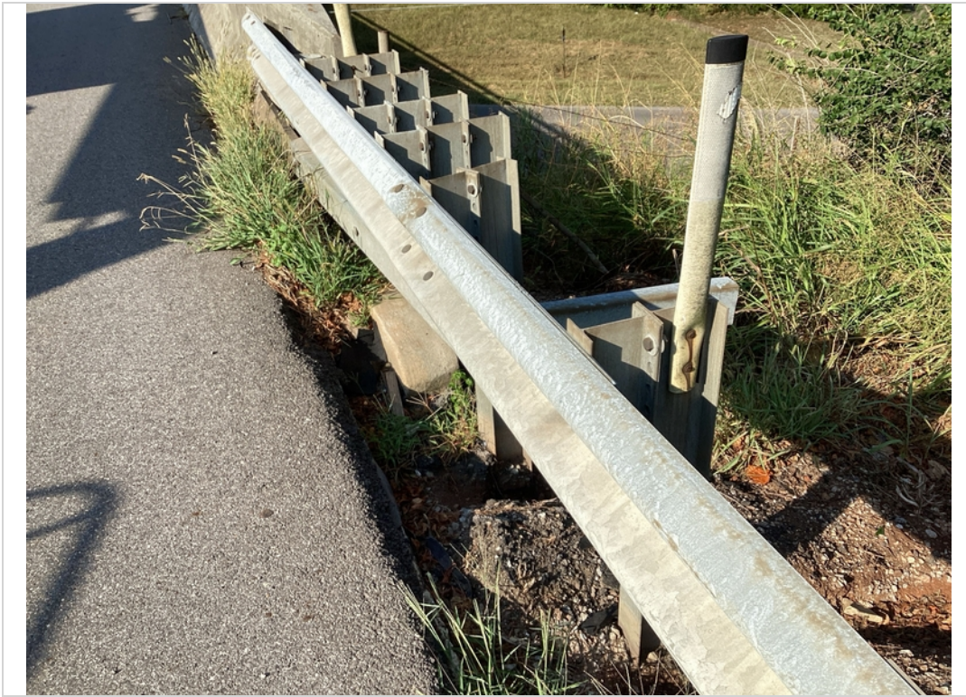
Approach 2 left embankment - moderate erosion ditches
