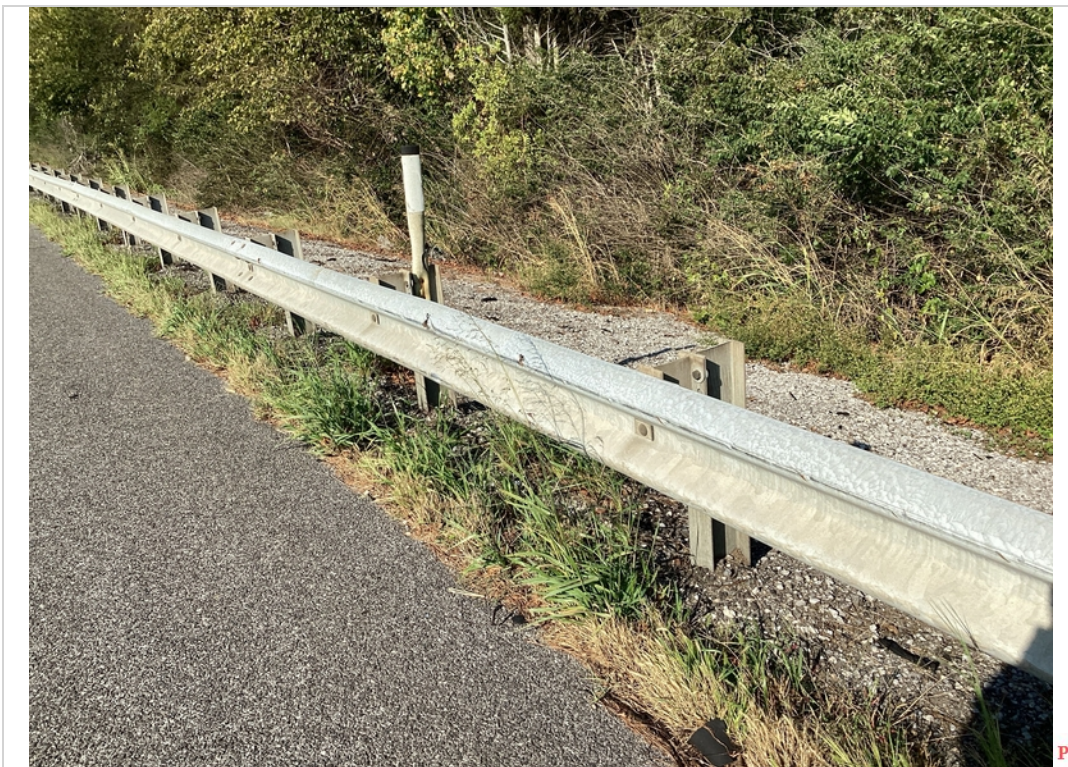
Approach 2 left rail - collision scrapes
