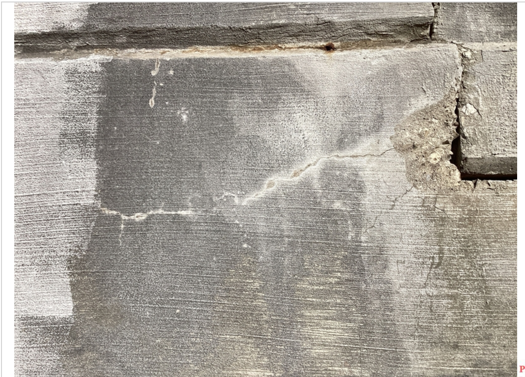
Wing 1 right - Hairline cracks with leaching - spall ( 4" diameter x 1/2" Dp)
