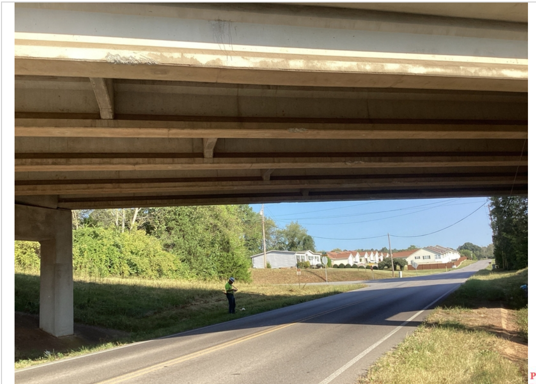
Beam A thru E right span 2 - Collision damage w/ scrapes & spalls up to 2' long 1" deep
