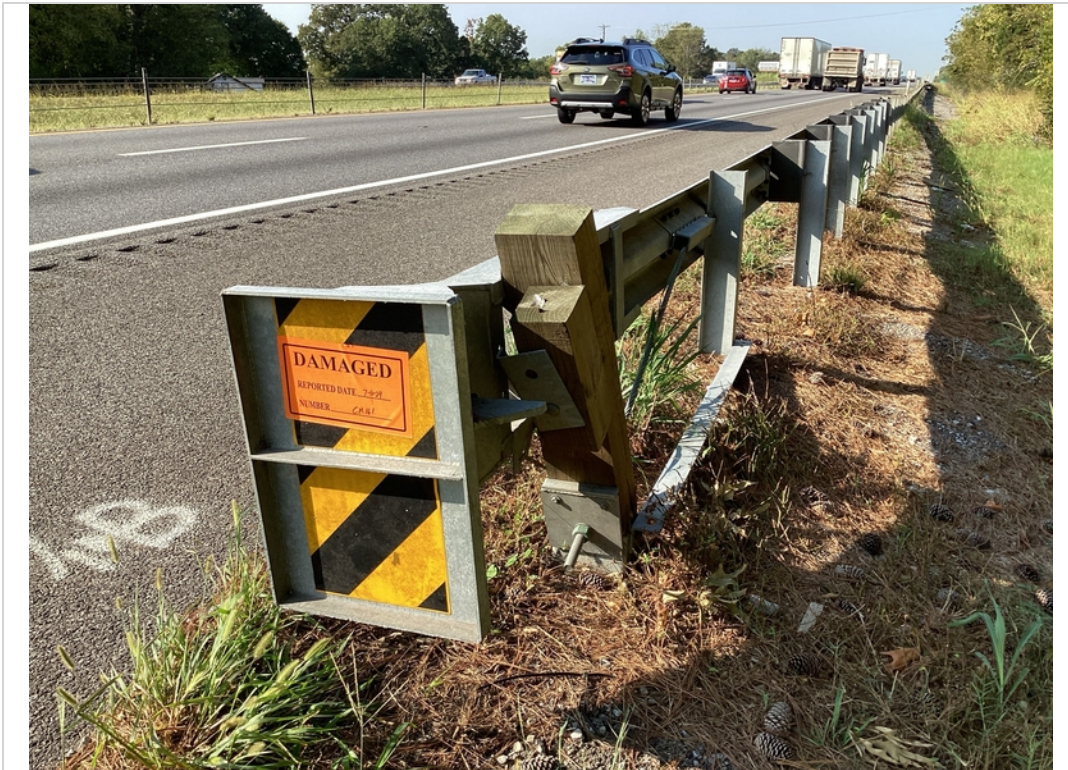
Approach 2 left rail - collision damage
